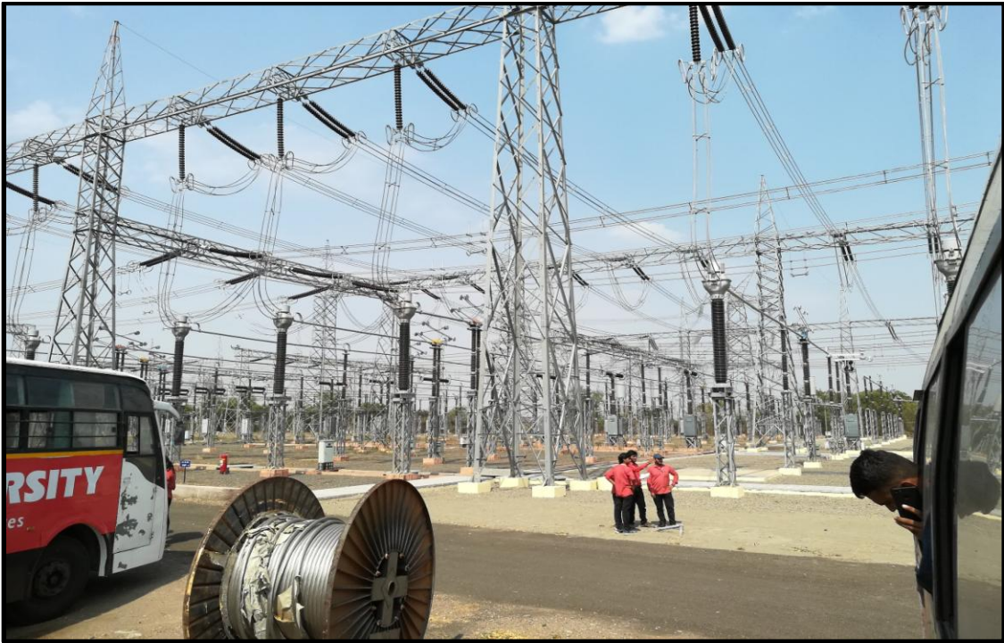
400kV Babhaleshwar Substation View
